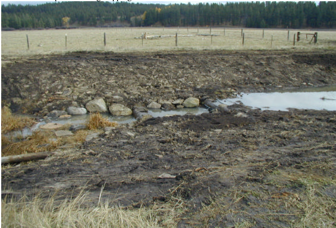
Figure 13. Bear Creek/Cunha Ranches, October 20, 2000. A completed set of weirs that has sealed up and is now running water over the tops. Banks have been sloped which will allow riparian vegetation to become established. However, this work is only a temporary fix, and in 2001 and beyond additional work will include reestablishment of a natural stream channel with constructed meanders, pools and riffles.
