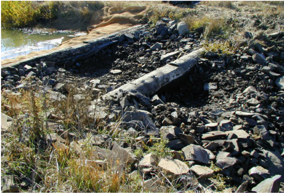
Figure 12. Bear Creek/Cunha Ranches, October 18, 2000. Jump pools were excavated behind log weirs to improve fish jumping ability. Coir fabric or geotextile cloth was trenched into the upstream faces of the structures to improve sealing/trapping of water.
